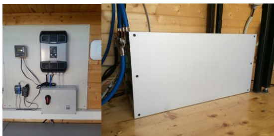
Figure 3: B2G setup. The grid-connected inverter/charger is shown on the left and the Lithium-Ion batteries on the right.
