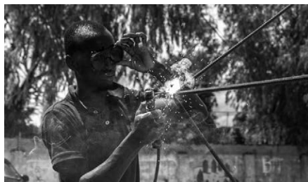
Fig. 5: A local welder man is giving the final touches to a Bantaba (garden pavilion) co-created by youth during the Weld Champions workshop in Soma.
